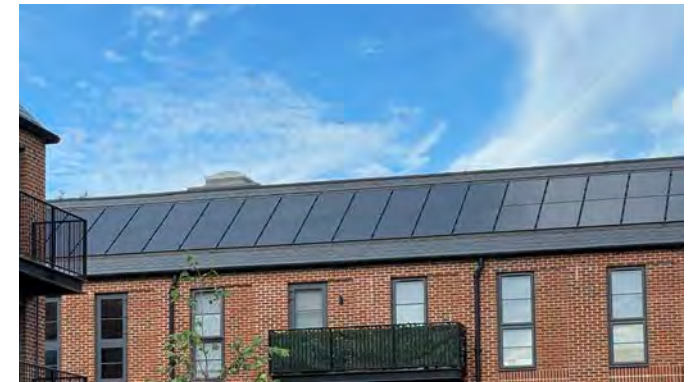
Flush photovoltaic panels incorporated into a roof
